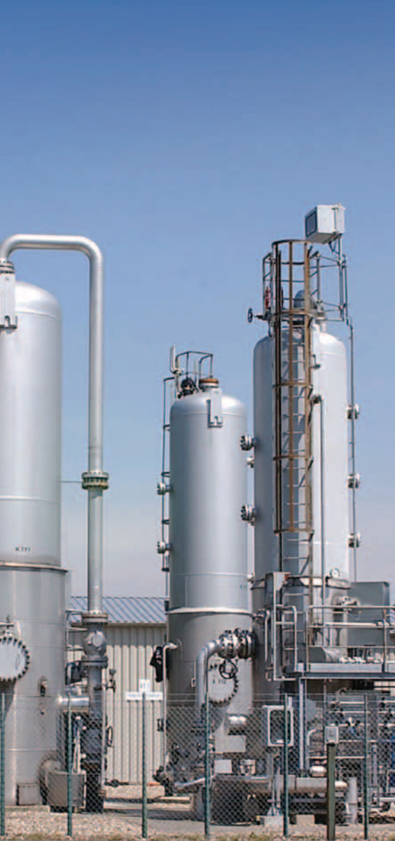
Gas storage facility Kalle, Germany, © RWE
